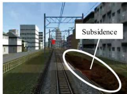
Fig. 2. Appearance of the subsidence
